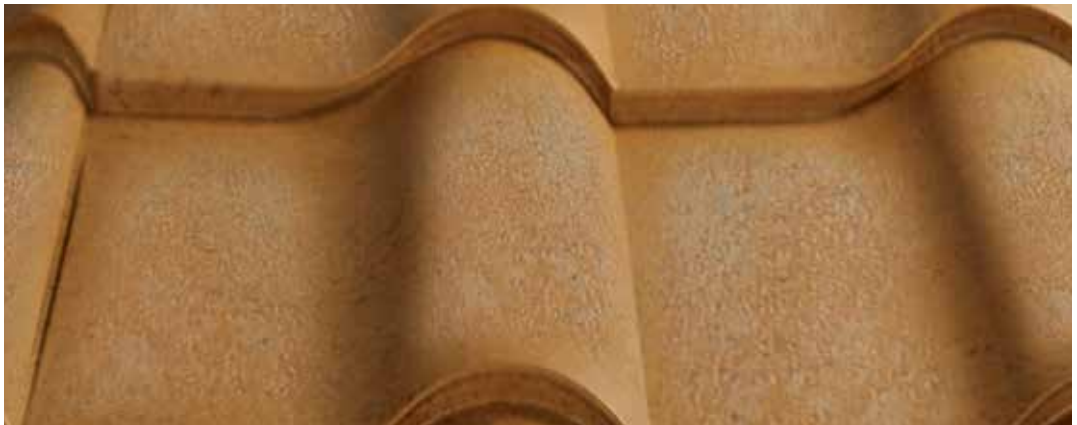
Weathered Terracotta CRRC# 0668-0111
